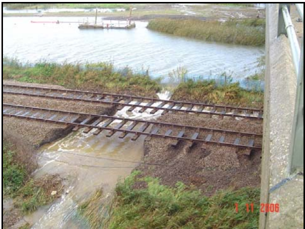
Breach at Haddiscoe Bridge
